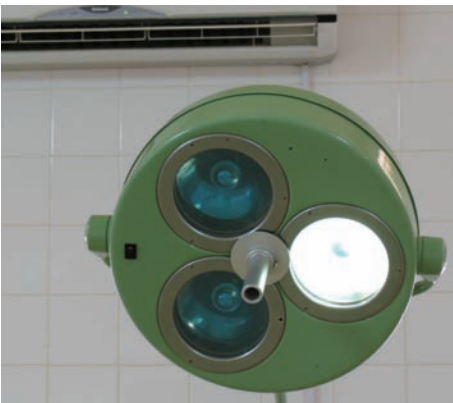
Figure 5.10 Faulty lighting equipment – a common situation in African hospitals.
